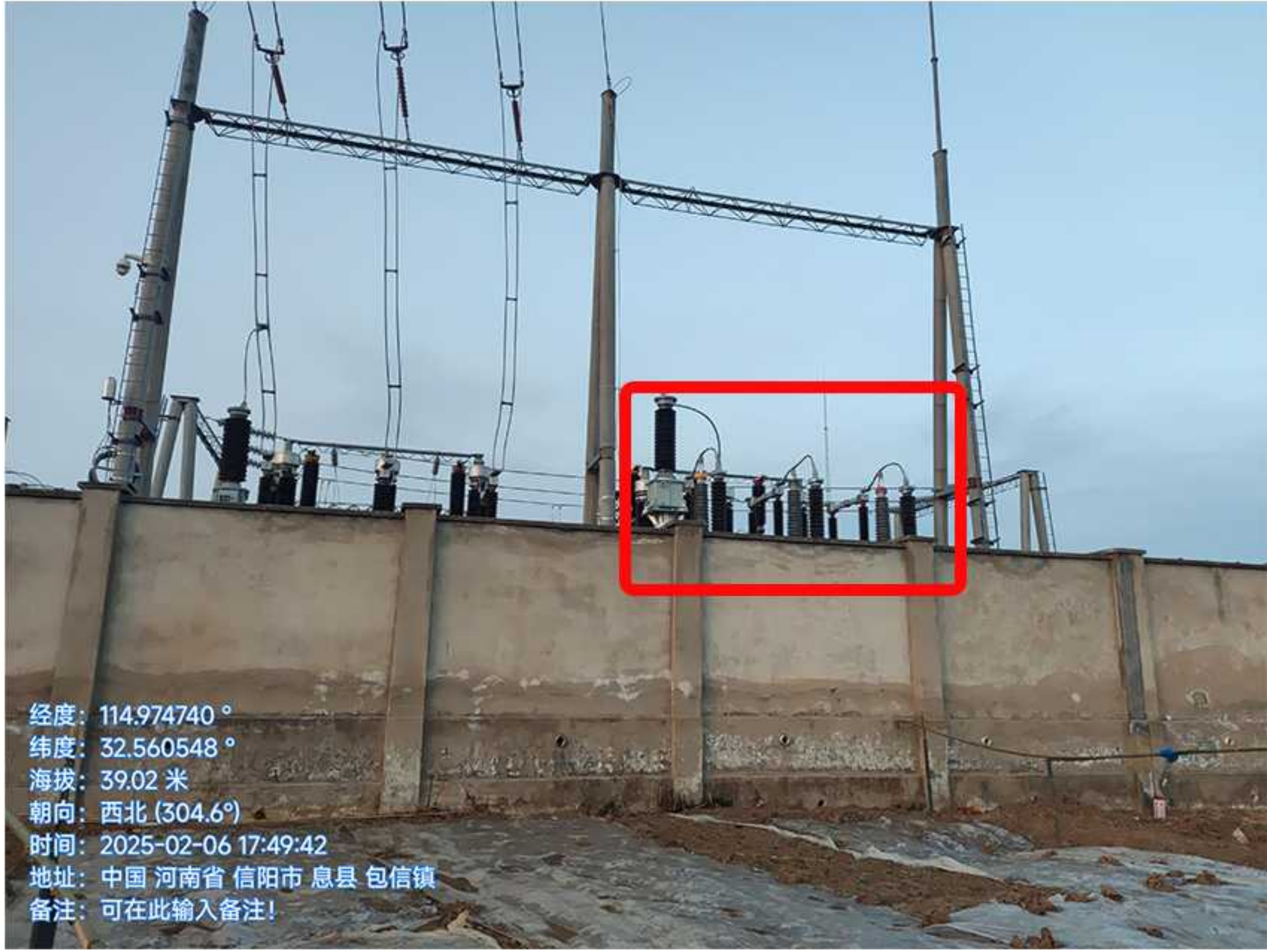
邹楼变出线间隔
